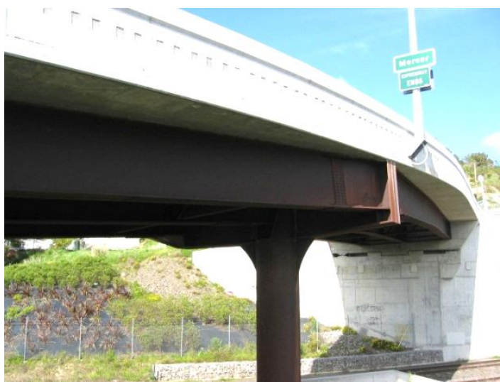
Figure 9.3: Mercer Bridge after four years weathering
