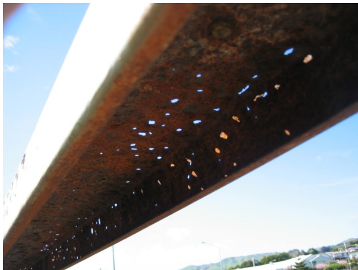
Figure 9.5: Inline galvanized purlin section used as handrail in marine environment
